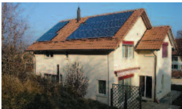
Installation photovoltaïque de 38 m²
